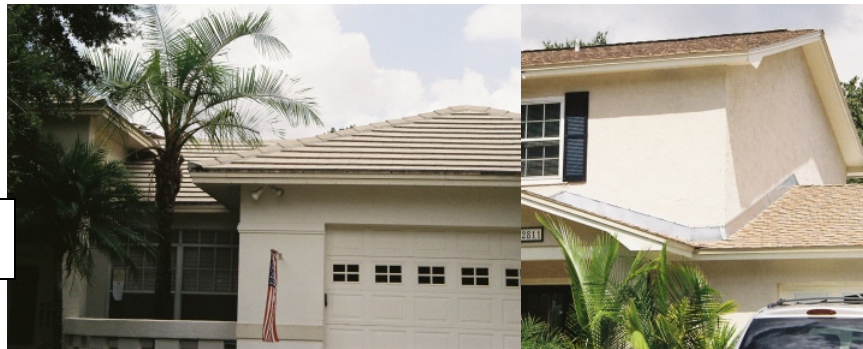
Unacceptable roofing: 20-year non-dimensional shingles. (Shingles are flat and have no shadow or thickness to them)
