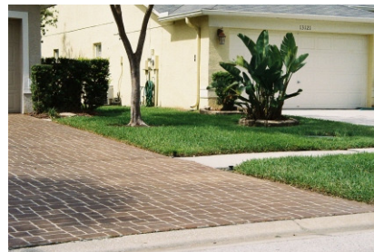
Unacceptable installation: paver material not flush with curb and street sidewalk. The paver material itself is acceptable.
